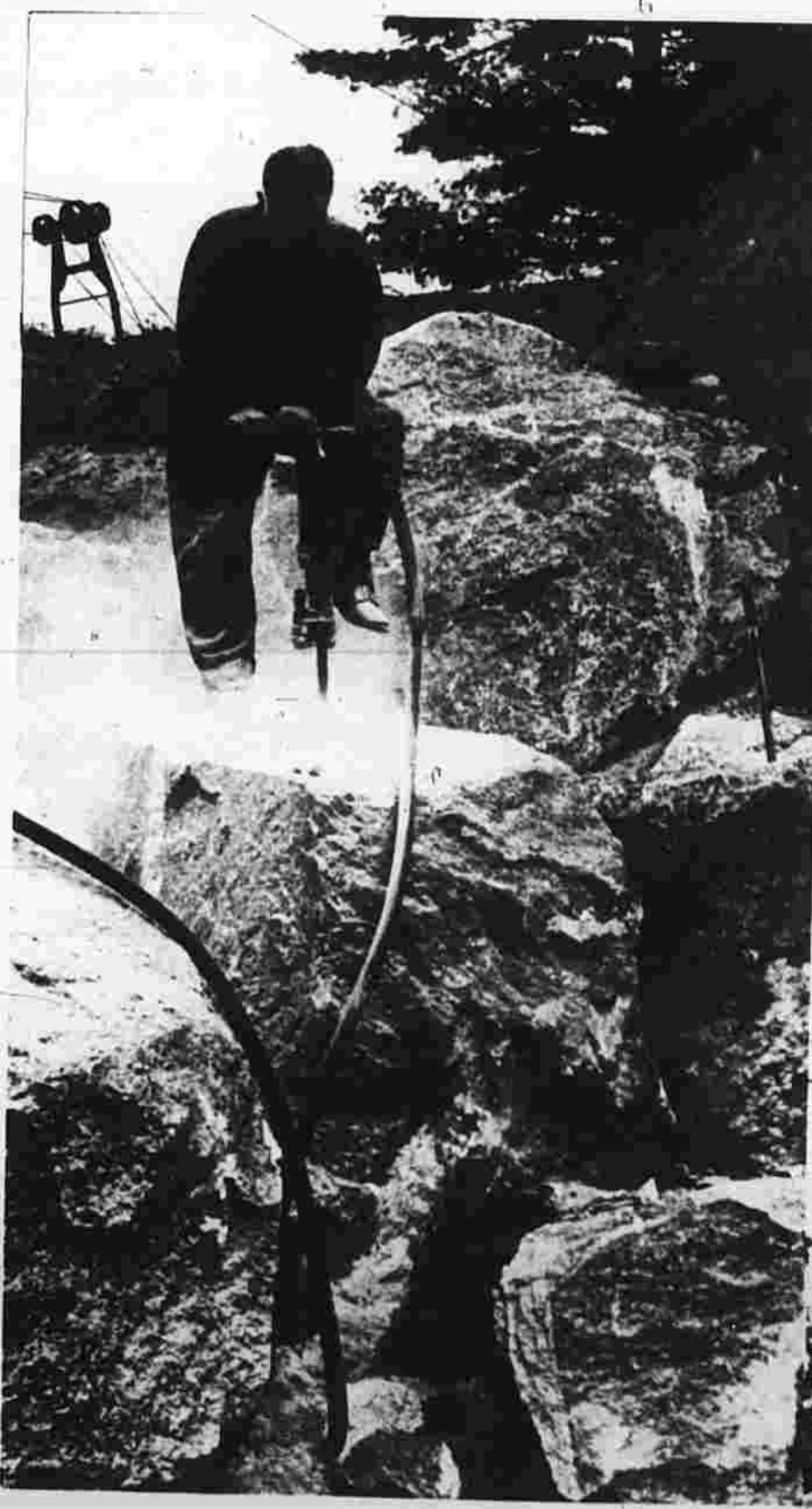
With part of a power shovel visible over a hill behind him, a worker begins to split a boulder.
